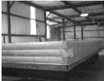
PowerLog Park Kabin Kottage log raising in a modern weather proof manufacturing facility.
